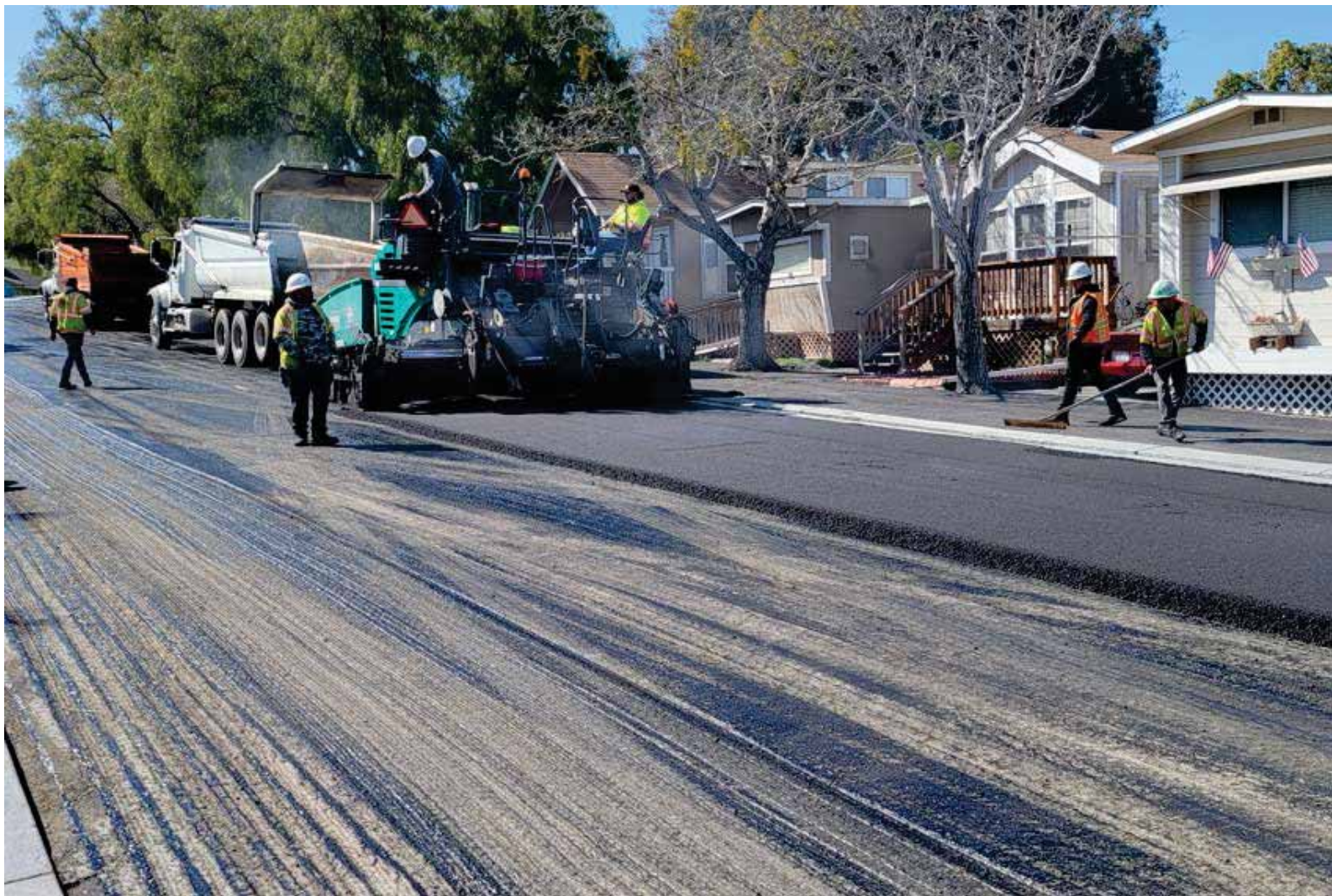
The Measure G funded pavement milling and overlay of Church Street in the City of San Juan Bautista.
