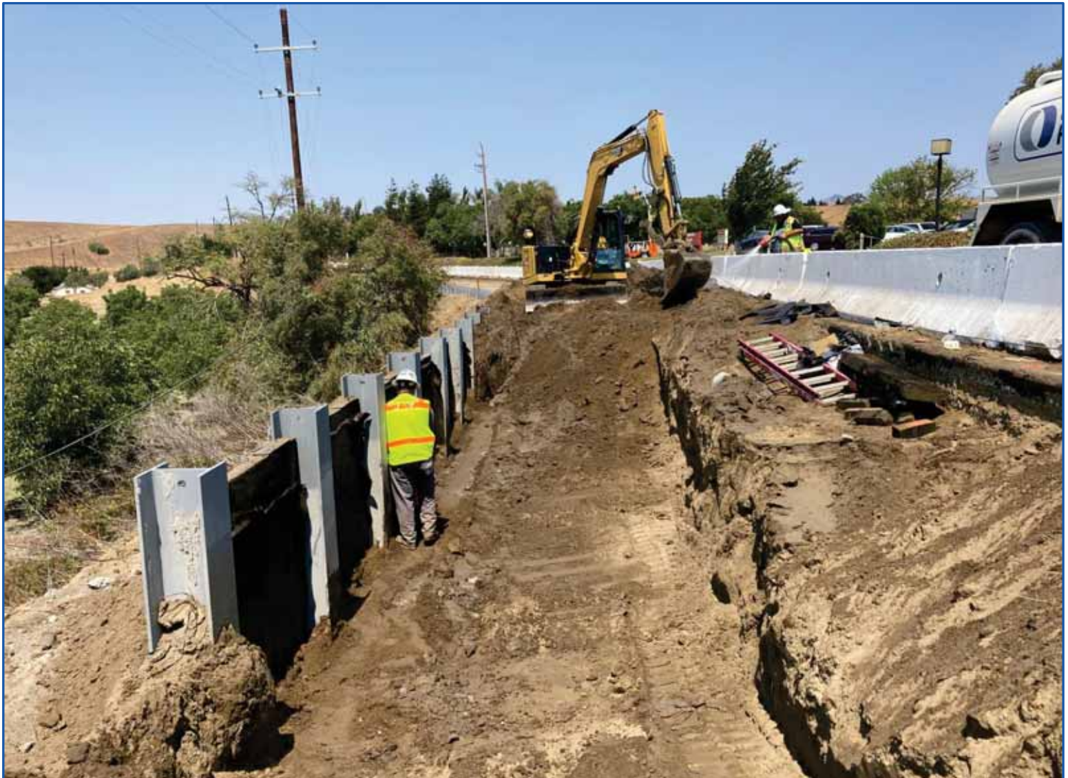
Construction and roadway excavation for the Measure G funded Southside Road – 5000 Block project.
