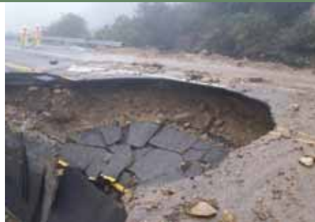
Landslide, Highway 154 in Santa Barbara County
