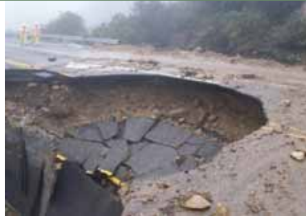
Landslide, Highway 154 in Santa Barbara County
